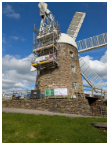
A general view of work in progress (picture by Roger Hatcher, October 2024)
