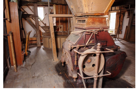
Inside Steinbeck Mill : before the cleaning of the 1st floor. Countless pipes, mixers, elevators, and grain storage facilities can be seen.
